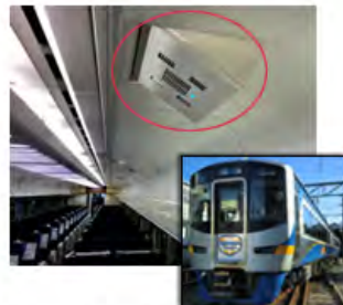
Plasmacluster ion generators are installed in the express trains of the Nankai Electric Railway Co., Ltd.
