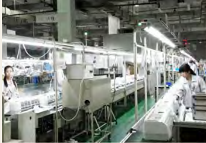
LED lighting installed above production lines
