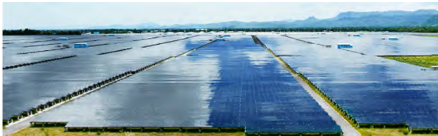
Mega-solar power plant in Lop Buri Province, Thailand
